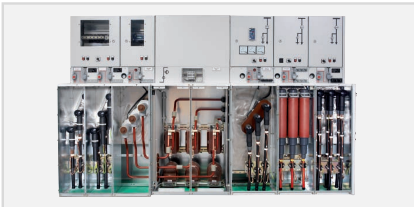
Combined customer-specific switchgear (front covers opened)
