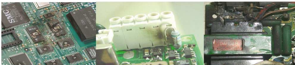
Burn-out of the electric devices due to surge
